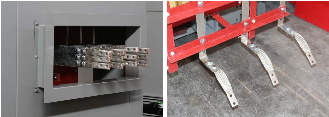
Figure 8: Low and High Voltage Terminals with Flexible Connectors, Coordinated to Mate with Adjacent Equipment
